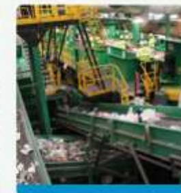
Refuse Separation Law for large refuse generators
